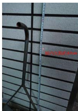
(c) 一樓地板沉陷約 47 cm
