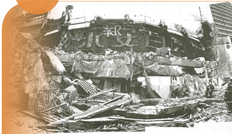
永安大廈在1994年拆卸期間倒塌 Collapse of the Wing On Building during demolition in 1994
